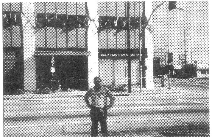
Figure 2 - Unusual 2nd story column failures resulted in building failure
